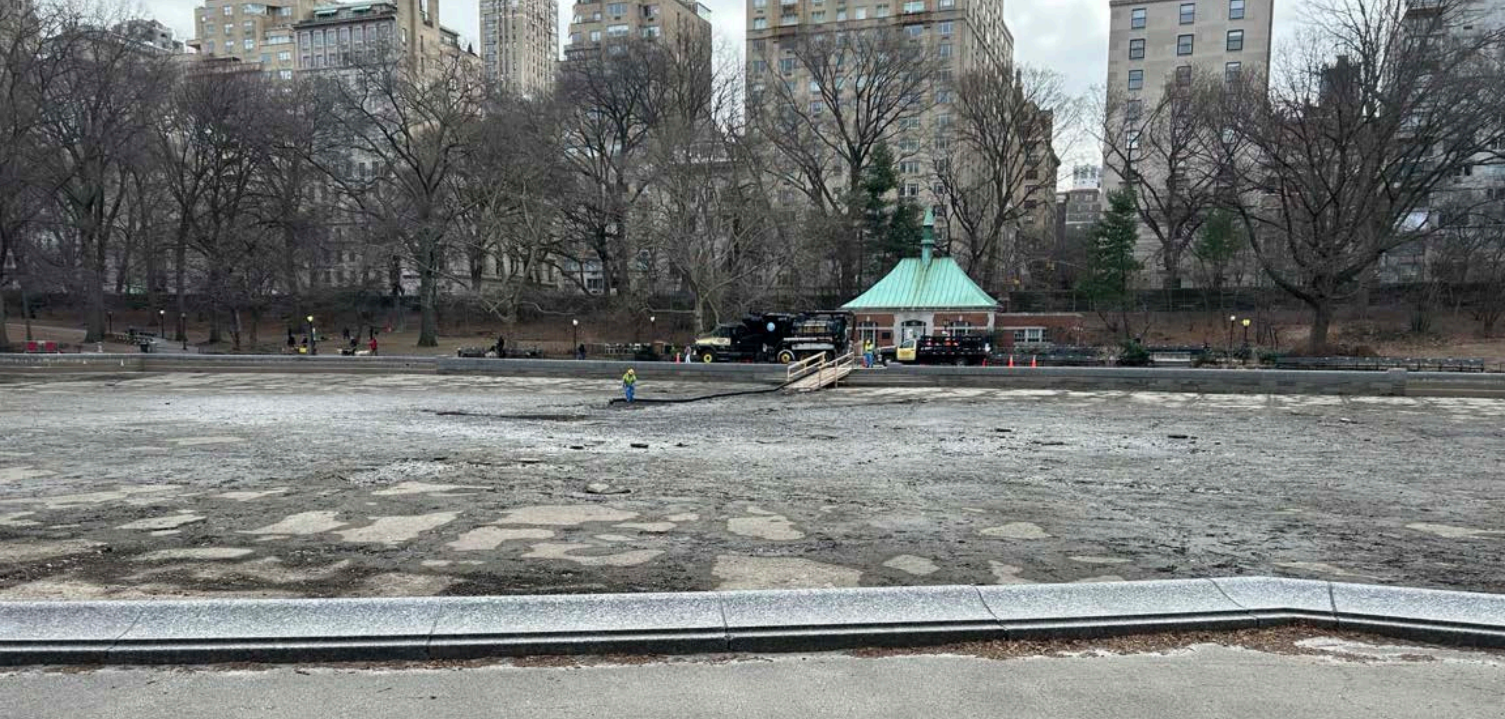
Conservatory Water Basin Floor, Existing Condition (Winter 2024)
