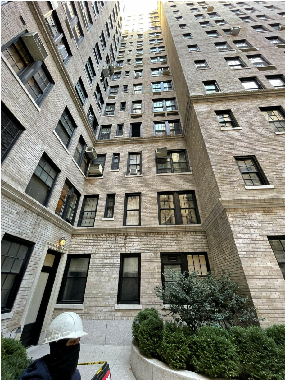
Existing Windows Condition - North Courtyard
