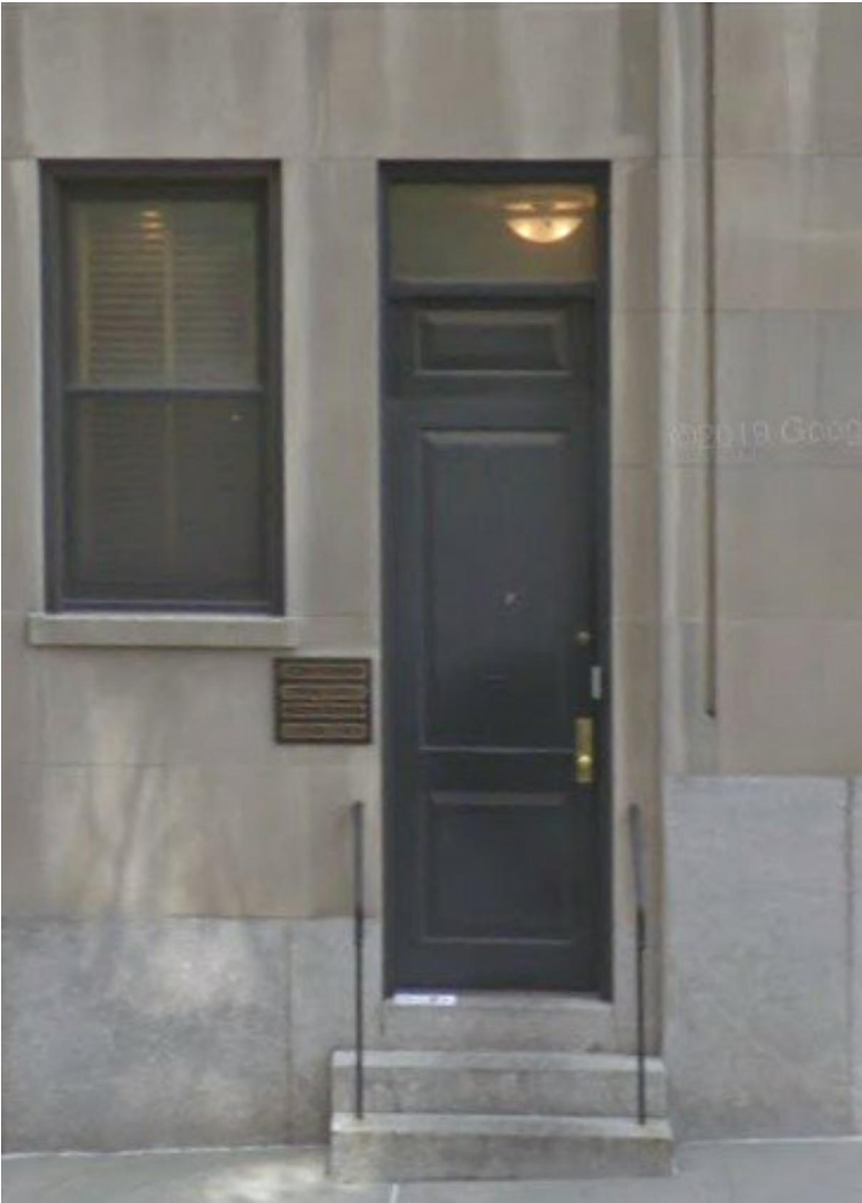
Existing Door Condition - Exterior View 10
