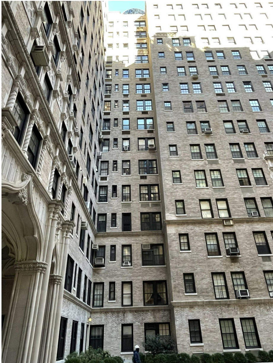
Existing Windows Condition - North Courtyard
