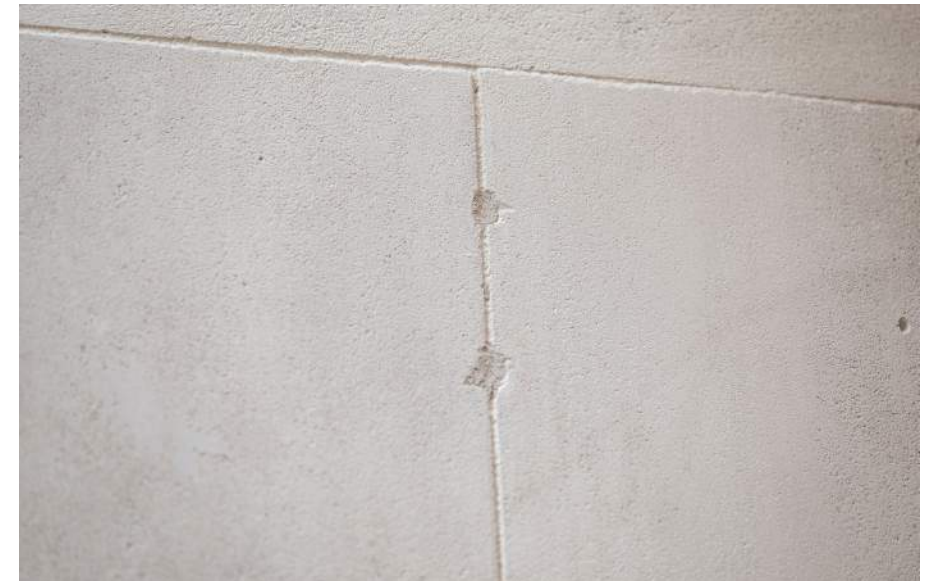
WALL DAMAGE & SUBSTANDARD REPAIR
