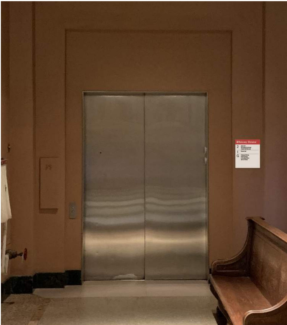
GREAT HALL, FIRST FLOOR FREIGHT ELEVATOR
