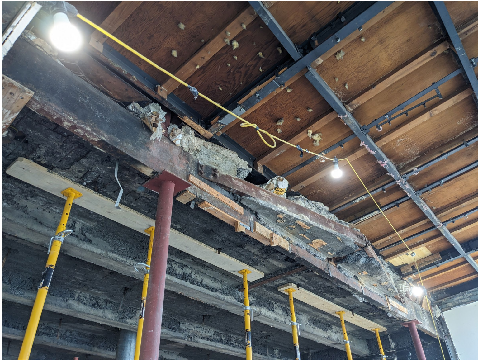
HISTORIC ROOF SLAB SEEN AT LEFT WITH ALTERED CONTEMPORARY ROOF STRUCTURE AT RIGHT.
