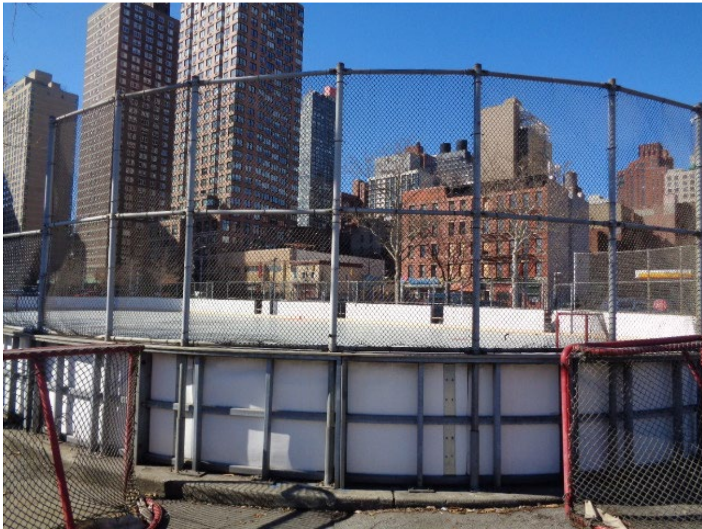
2 – Walls and chain-link fence to be replaced
