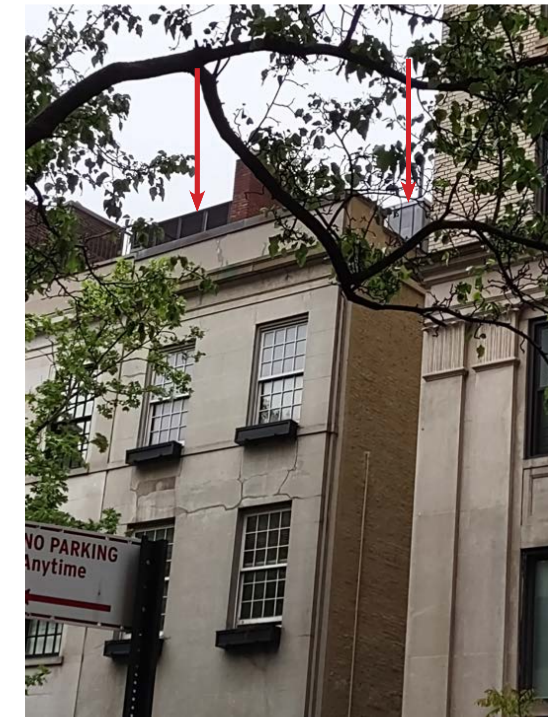
63 AND 65 EAST 92ND ST. ZOOMED IN. VIEWED WALKING EAST. ROOFTOP ADDITIONS ARE VISIBLE (MAY 2023)
