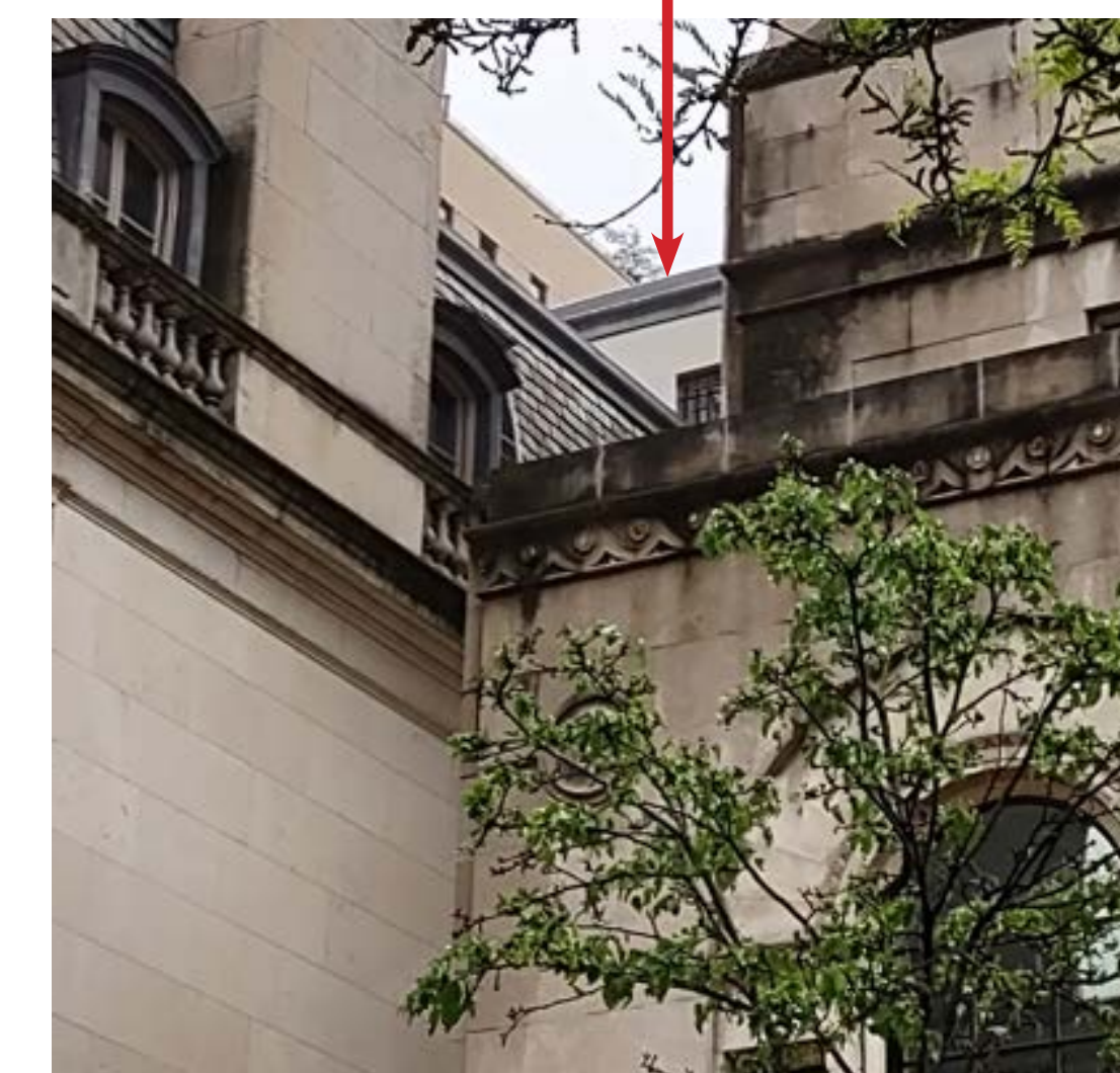
60 EAST 93RD ST. ZOOMED IN. VIEWED FROM ACROSS THE STREET AND WALKING WEST. ROOFTOP ADDITIONS ARE VISIBLE (MAY 2023)
