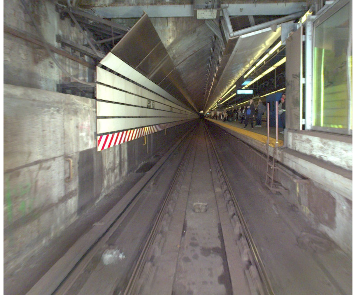
Above: Deteriorated direct fixation track at Lexington Av/63 St
