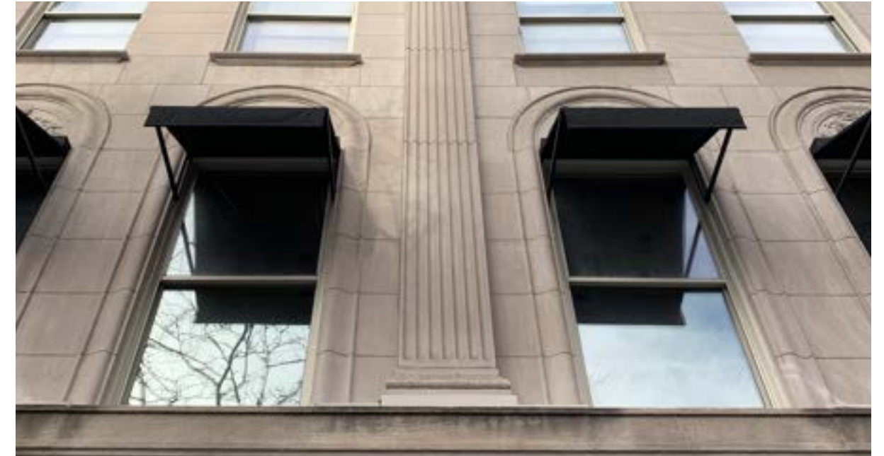
EXISTING DOUBLE HUNG WINDOW Typical @ 2nd and 3rd Fl To be replaced with new bronze type at 2nd Floor - 21 total units
