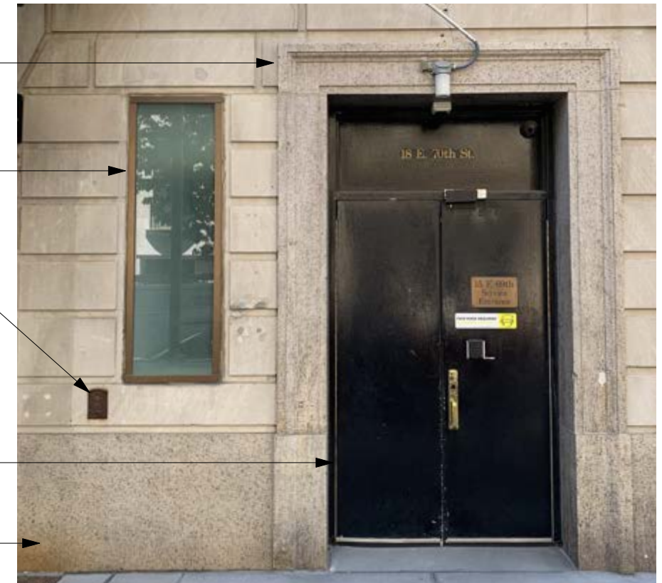
EXISTING PARTIAL E70TH STREET FACADE Existing commercial window and pair of residential egress/service doors; Window to be altered to new 36" wide egress/service door for commercial space - see sheet 9
