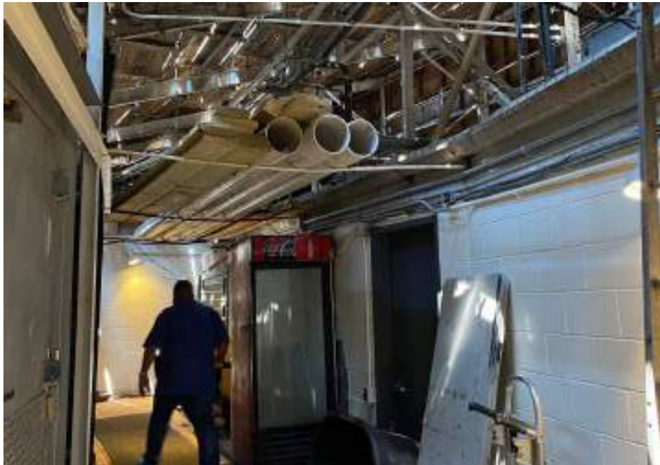
View of Deteriorating Conditions (Inefficient Work Areas) 2021
