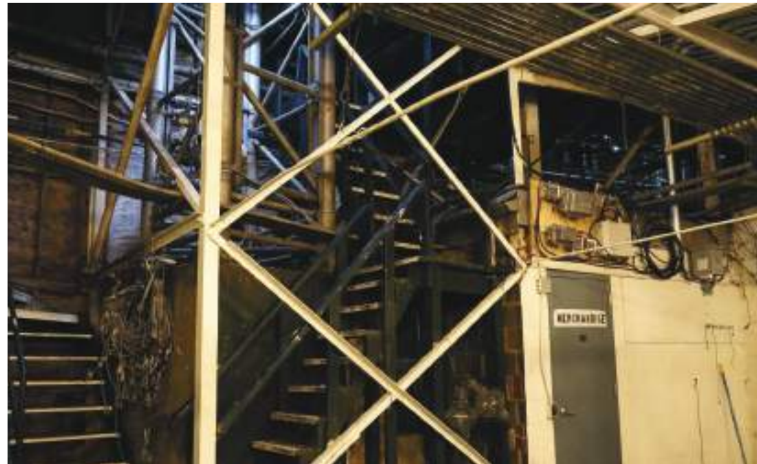
View of Deteriorating Conditions 2021
