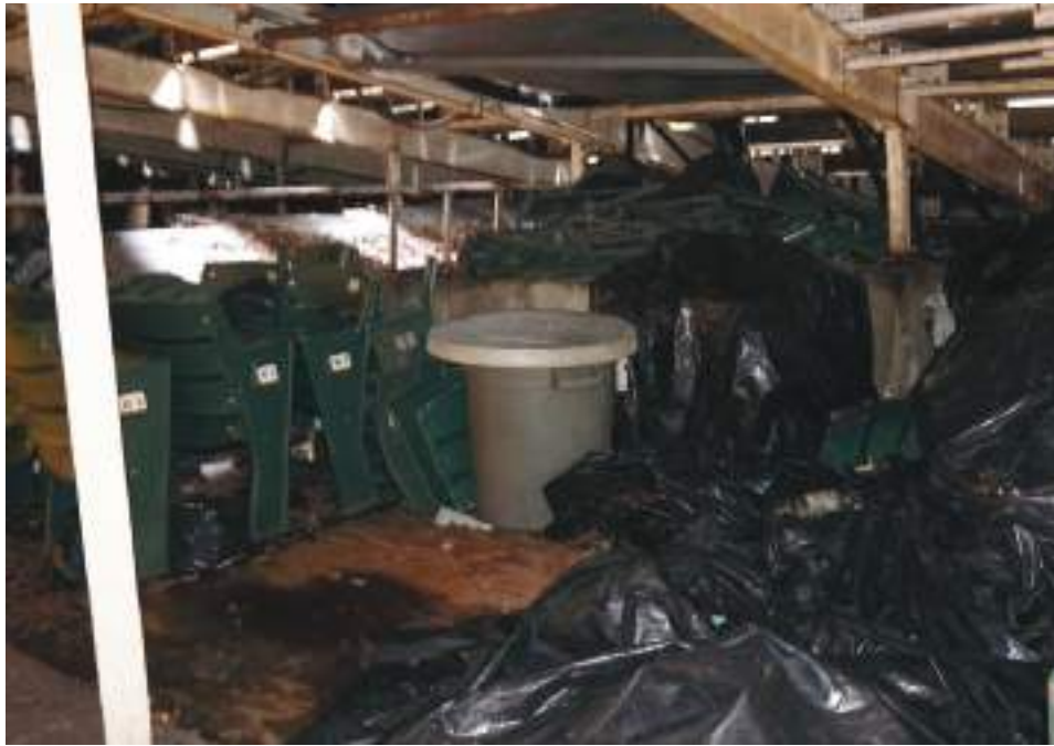
View of Deteriorating Conditions (Improvised / No Waterproofing) 2021
