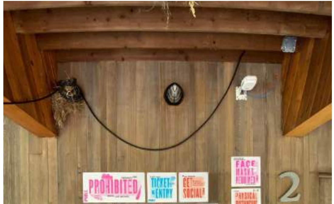
View of Deteriorating Conditions 2021
