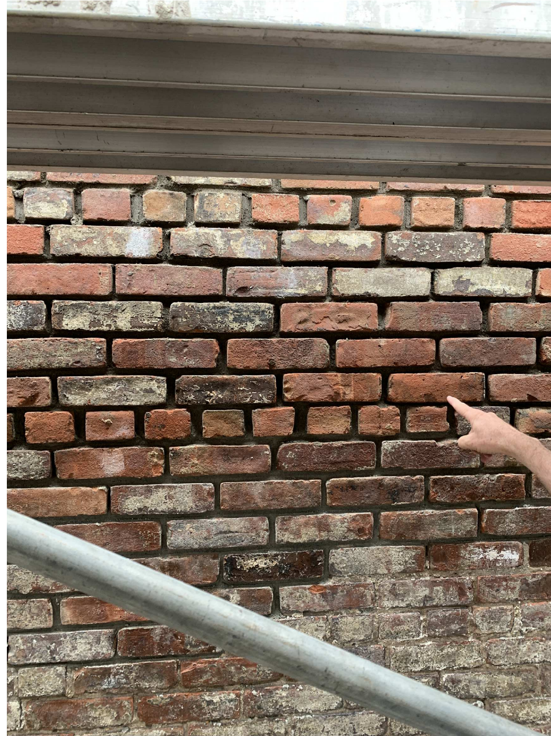
PHOTO SHOWS BLENDED MIX OF NEW AND EXISTING (SALVAGED) BRICKS AT CURRENT REPAIR WORK ON THE NORTH WALL. THIS SAME BLENDED MIX OF NEW AND SALVAGED BRICKS PREVIOUSLY APPROVED FOR PATCHING AND REPAIRS ON THE NORTH ELEVATION IS PROPOSED FOR USE AT THE ELEVATOR BULKHEAD.
