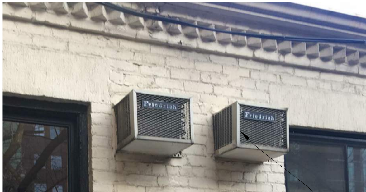
EX'G THRU-WALL AC UNITS
