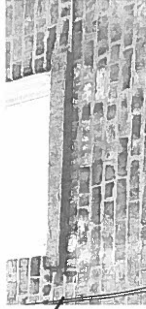
EXISTING WINDOW CONDITIONS IN DISREPAIR
