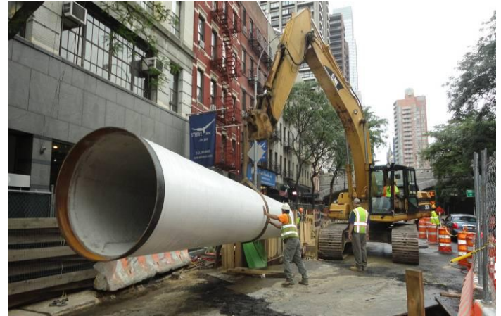
Workers prepare to install a section of the 48-inch trunk water main on E. 59 th St. between 1 st Ave. and 2 nd Ave.
