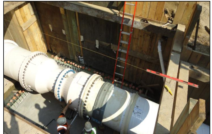
Workers install a Venturi flow meter on E. 59 th St. between 1 st Ave. and 2 nd Ave. The Venturi meter, which connects sections of the 48-inch trunk water main, measures the flow of water through the trunk main.
